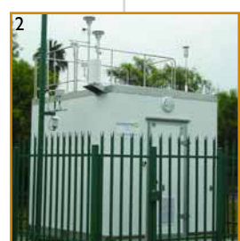
1. Air Quality Analyzers 2. Air Quality Monitoring Station
